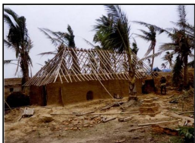
Figure 14 : Damage caused due to cyclone in Orissa
