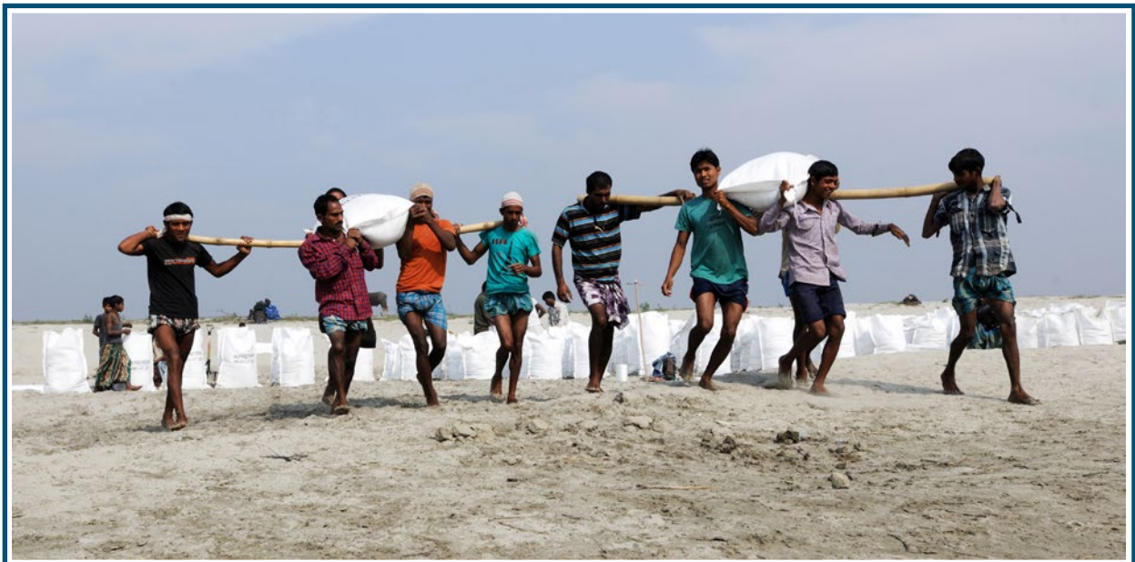
Workers carrying sand filled geo bags to be pitched on the banks of the river Brahmaputra in Gumi village, Guwahati as part of the Assam Integrated Flood and Riverbank Erosion Risk Management Investment Program. Photo: Rakesh Sahai for ADB
